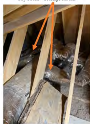
ITEM #5 Undersized ducts Toy room / Storage Room
