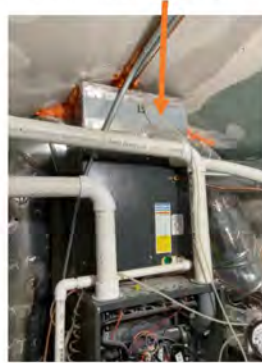
ITEM #1 Restrictive Supply Plenum
