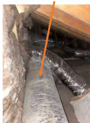
ITEM #4 Supply Trunk undersized
