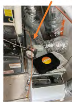
ITEM#2 Restrictive Return Air Drop
