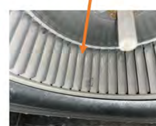
ITEM #6 Blower Wheel dirty
